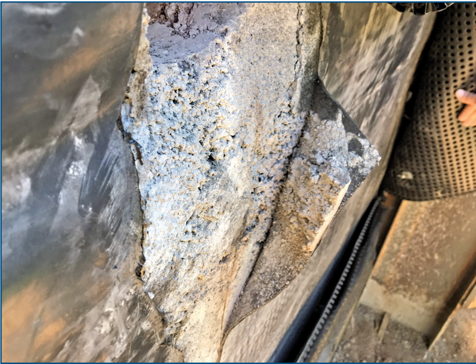
Figure 6 – Full-scale stand-alone mock-up at poorly consolidated shotcrete and overspray.
